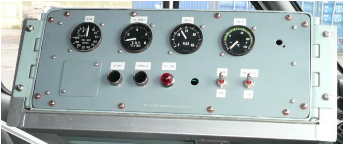
Simple instrument panel incorporating starting controls and indicators
